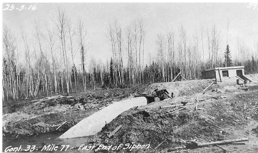
Figure 8.7.7.2. One end of a finished siphon showing the vertical curve and the housing of adjacent overflow structure (GWWD No. 391)
