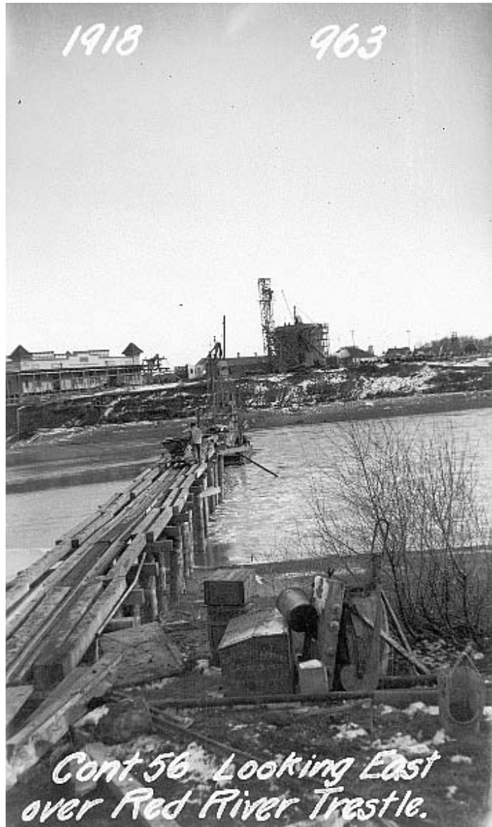
Figure 8.10.2 Trestle on Red River with concreting tower and surge tank in background (GWWD No. 963)
