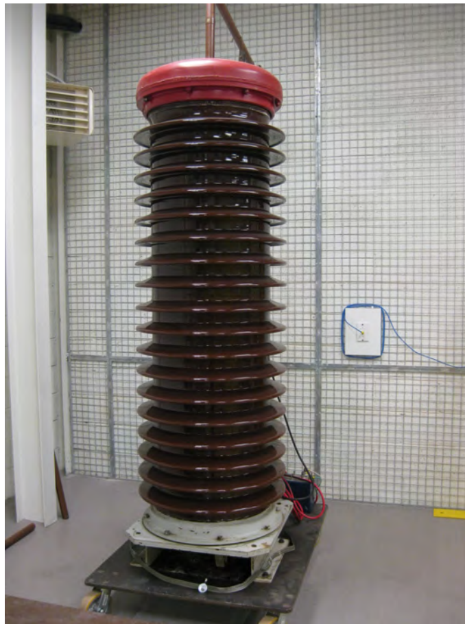
Figure 4.2: 230 kV potential transformer.
