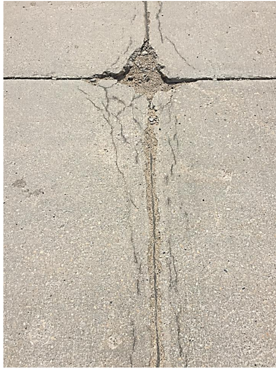
Figure 2.4- A sample of premature deterioration of joint in concrete pavement showing trapped water in developed microcracks parallel to the joint.
