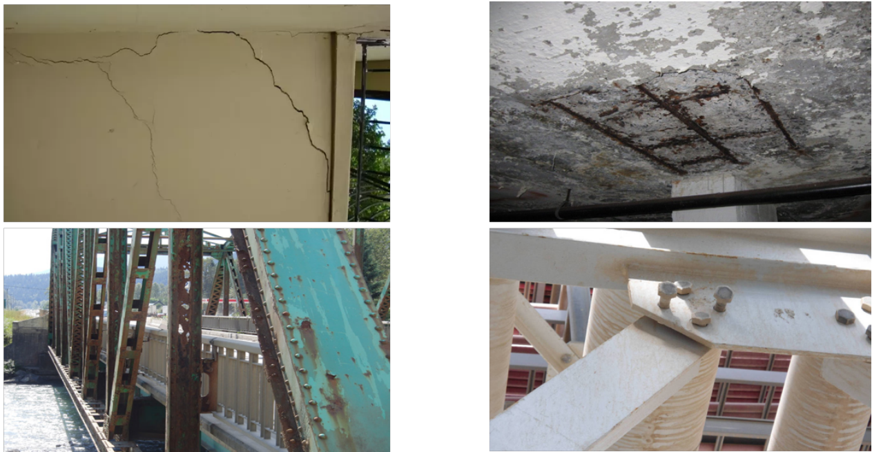
Figure 2.1. Types of defects in civil structures
