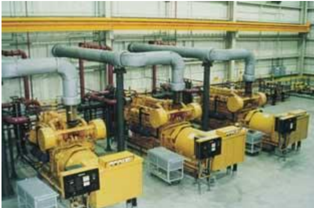
Figure 3-8: Existing Diesel Generators at Brochet. Source: Poweronline.com, 2000
