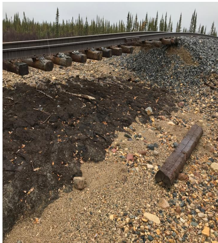
Figure 2 2017 Churchill Railway Washout
