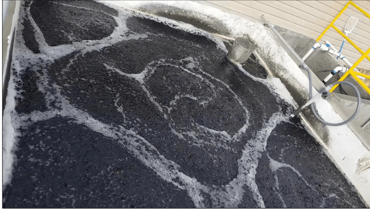
Figure 2.3: Working MBBR – Courtesy of Nexom (Nexom, 2021a)
