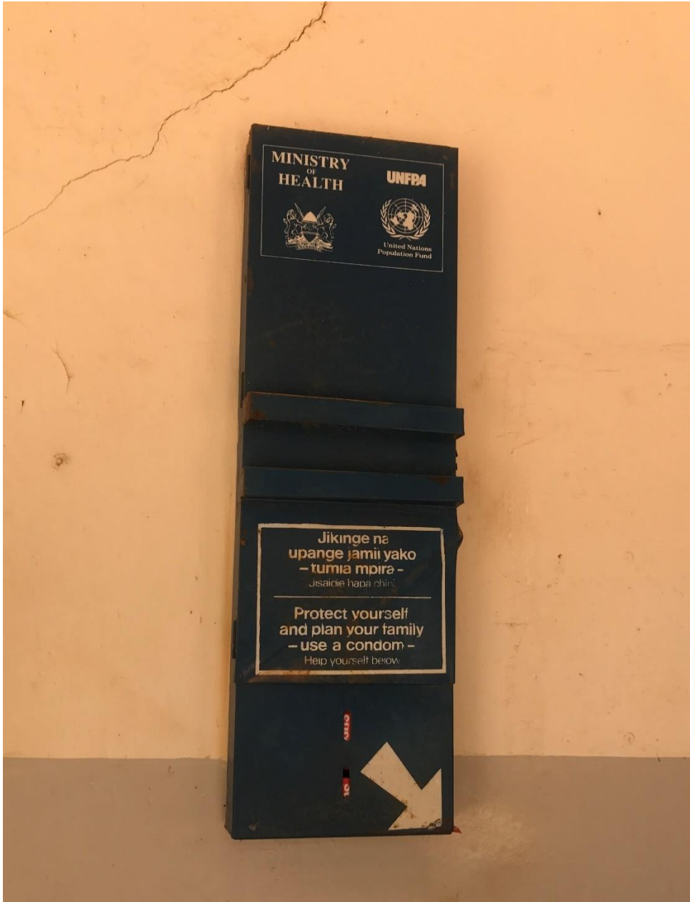
Figure 13. Condom dispenser on the cracked wall of a healthcare facility in Wundanyi. These dispensers can be found on the walls of almost every healthcare facility in the county, although the majority seem to be empty now.
