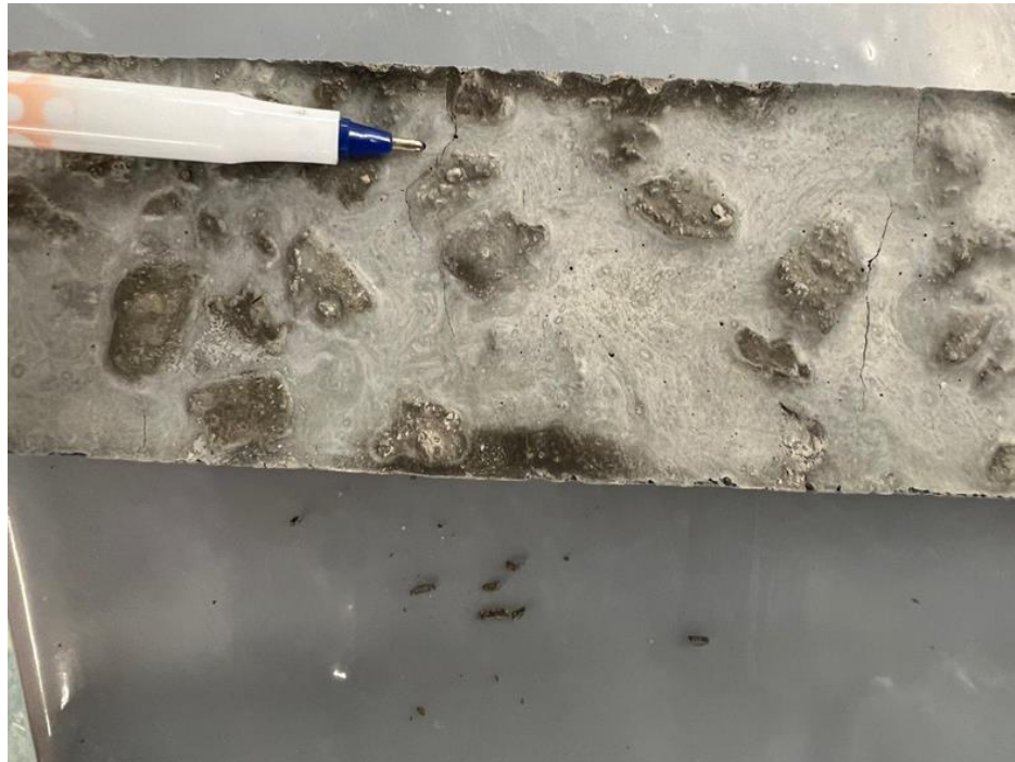
Figure 6.7: Thermal stress and surface cracking.
