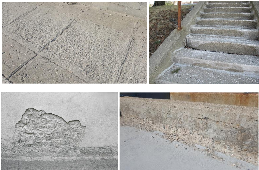
Figure 2.1: Effect of freezing and thawing on concrete (Sacco 2014; Fritz 2019; Saha 2019).
