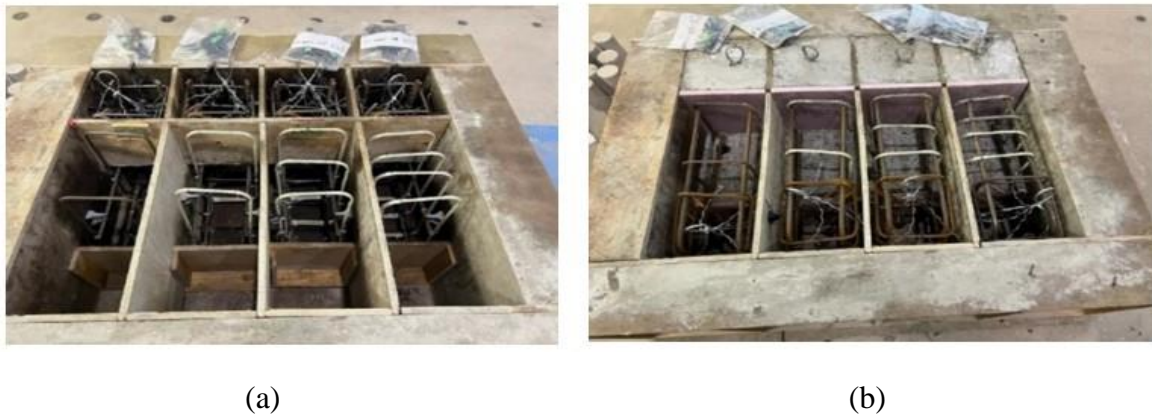
Figure 3.2: Casting stages, (a) reinforcement for first L-block with the intended connectors, and (b) reinforcement for the second block
