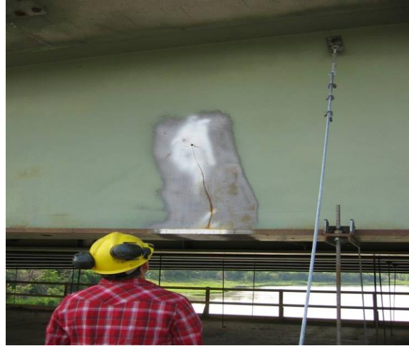
Figure 6-4: Crack in an inner girder of the PBX
