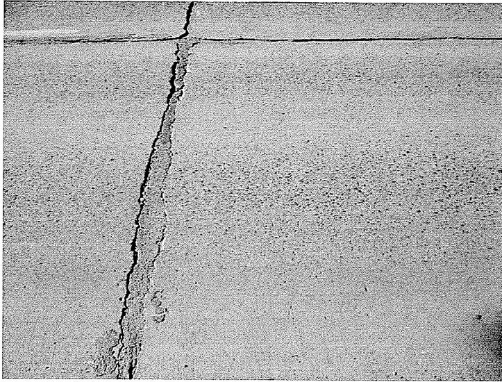
Figure 3.10: A spalled joint on Grant
