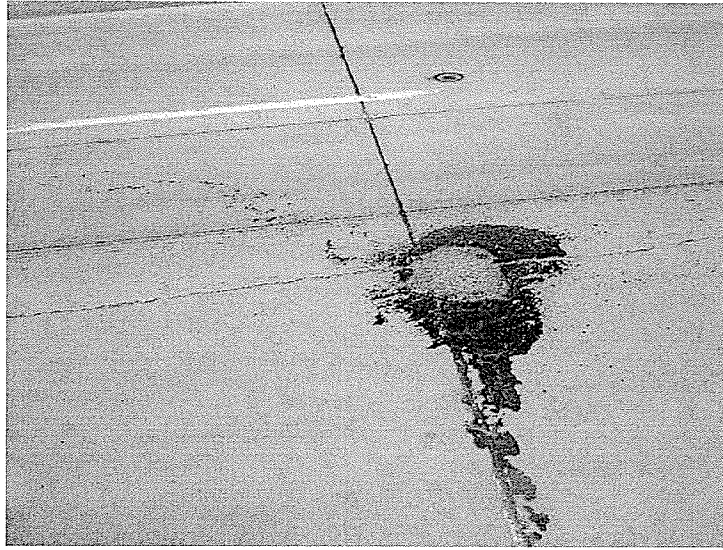
Figure 3.12: A spalled and patched joint on St. Mary's
