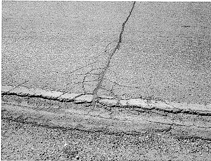
Figure 3.11: A spalled joint on Fermor
