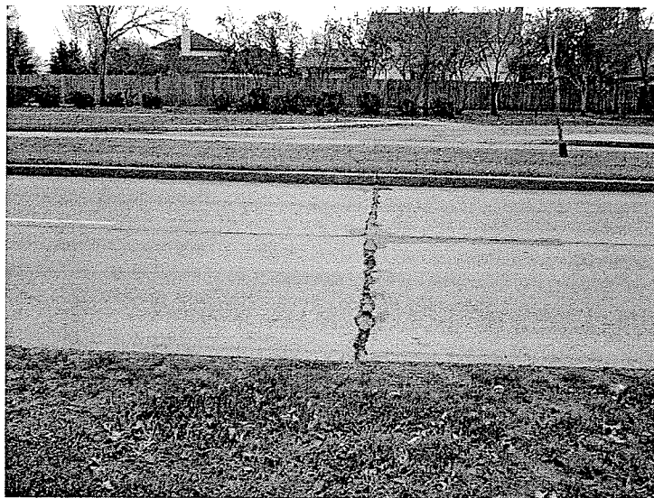
Figure 2.4: A spalled joint filled with patching material
