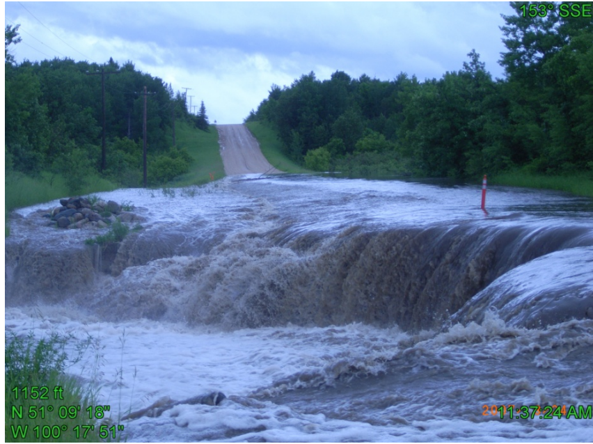
Figure 3.4 –Mile Road 121W During June, 2013 Flood Event (South from Ashville Junction)
