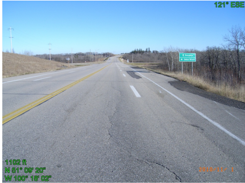
Figure 1.4 – November 2010, Progression of Pavement Cracking in EBL
