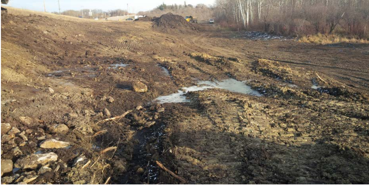
Photo 16 – Seepage from Slope Face at Mid-Slope
