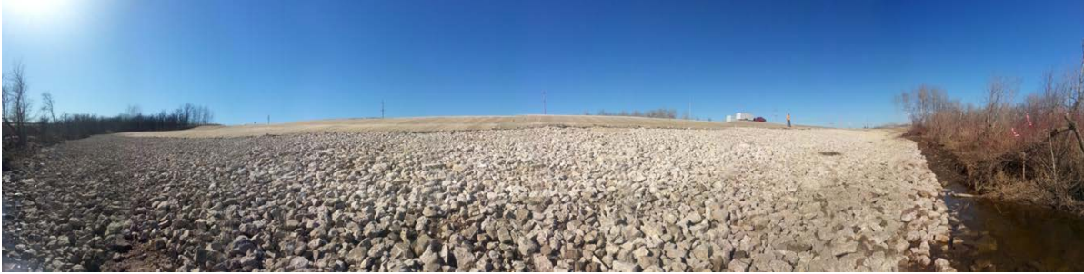
Photo 25 – Berm at Design Grade Following Rip Rap and Erosion Control Blanket Placement
