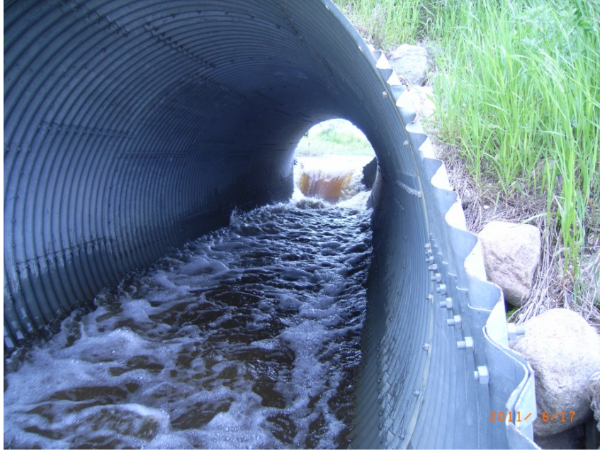
Figure 3.6 – Corrugated Steel Pipe Culvert Crossing Outfitted with Weir During Normal Flow Conditions in June, 2011 (West from outlet)
