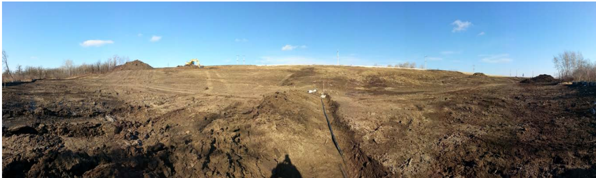
Photo 17 – Compaction Prior to Fill Placement (Conduit for Instrument Relocation shown in Centre)
