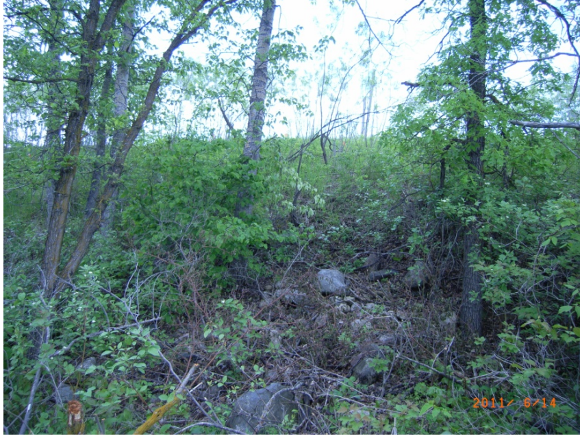
Figure 3.1 – General Terrain of Grade Slope at PTH 5 (North from mid-slope at station 185+70)
