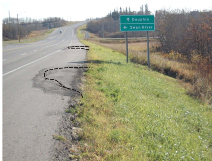
Figure 1.3 – October 2007, Shoulder Slumps in Shoulder of EBL
