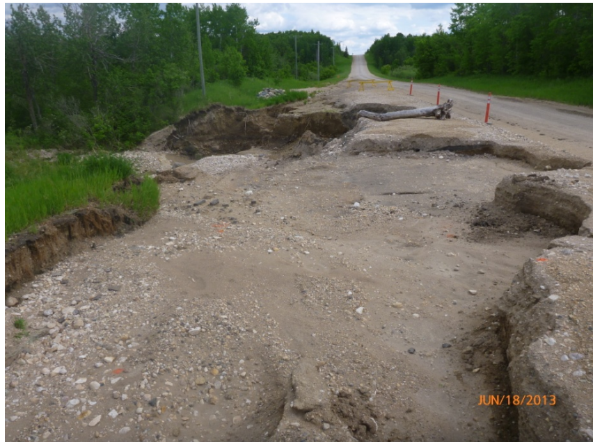
Figure 3.5 – Washout of Mile Road 121W Following June, 2013 Flood Event (South from Ashville Junction)
