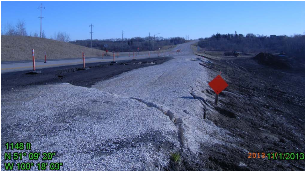
Photo 15 – Slope Movements Following Clearing and Grubbing
