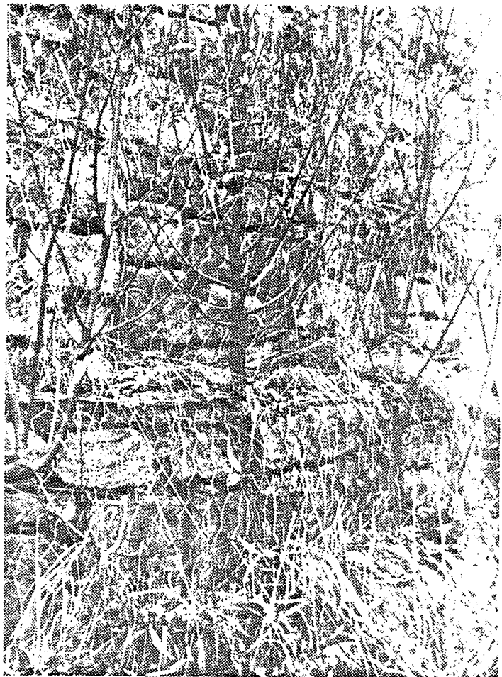
Figure 67 Gabions consisting of a rock pile wrapped in wire mesh, vegetated with live branch layering. If large rocks are used, the branches can be placed only in the joints between the individual gabions.
