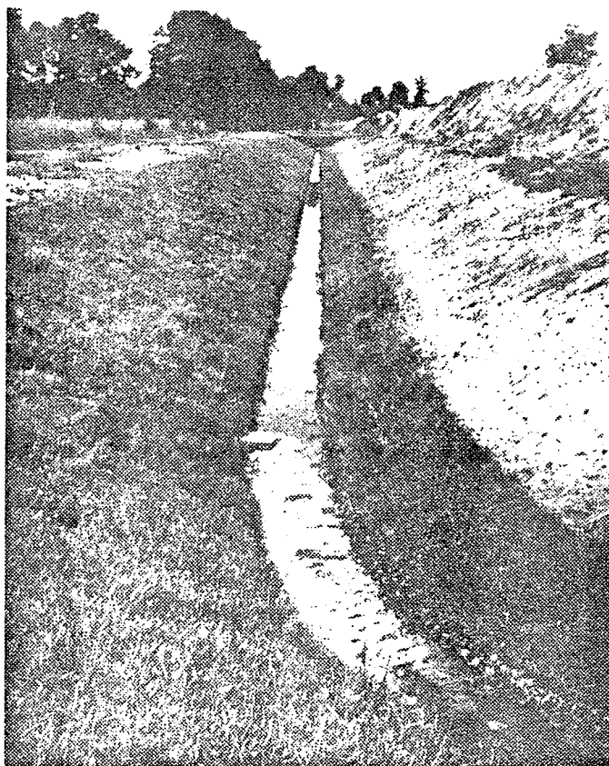
Figure 32 Sod slabs obtained while excavating ditch are placed in strips on the most critical sections of the slope.
