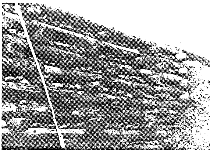
Figure 62 Crib wall as temporary stabilization construction. The gaps are filled with rocks. If long durability is required the gaps must be filled with live branches of woody species or rooted plants.
