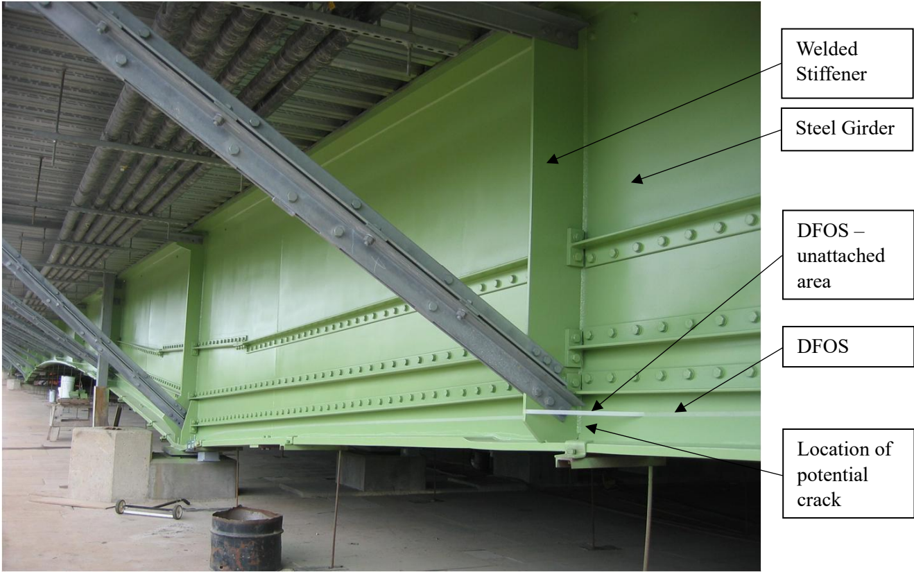
Figure 1.1: Steel girder with welded stiffener and FOS in a current monitoring system
