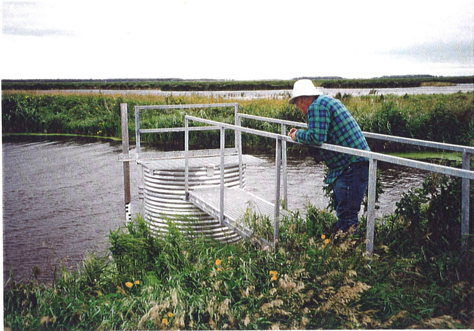
Figure 2.5. A stop-log structure located at the Duck's Unlimited Lynch Point Project site permits precise manipulation of water levels.
