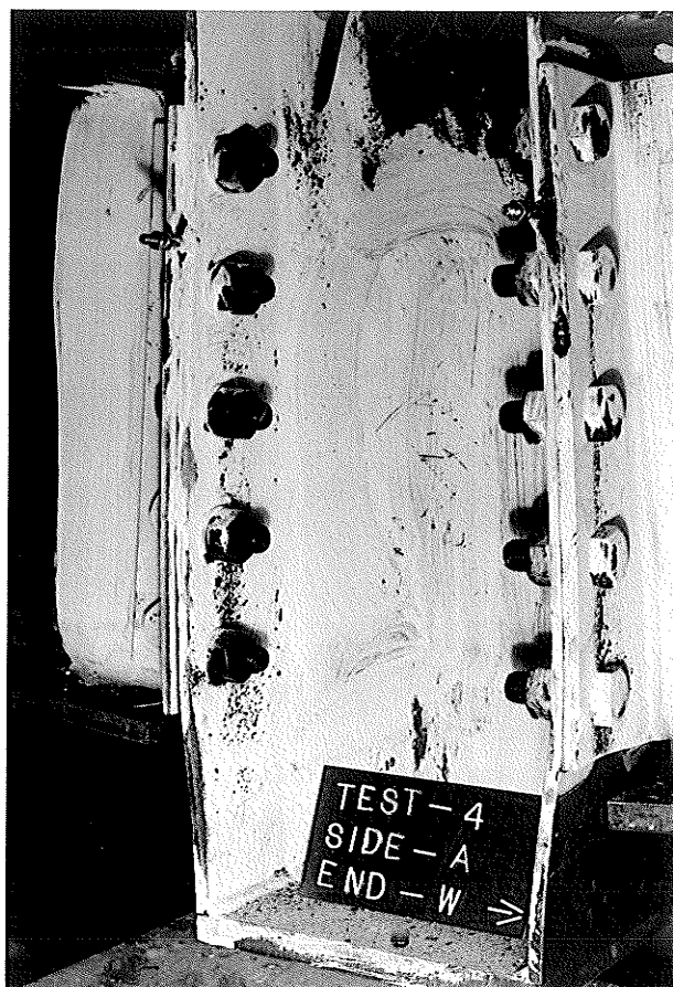
Figure 5.33: Deformation of Both Column Flange and Web in Specimen 4.
