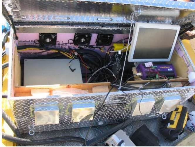
Figure 46: On-board control cabinet housing instrumentation and data conditioners.
