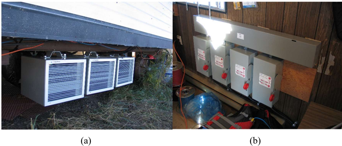
Figure 78: (a) Unit heaters used as resistive loads, mounted below U of M trailer (4th unit behind not shown), and (b) splitter and switches located in trailer.
