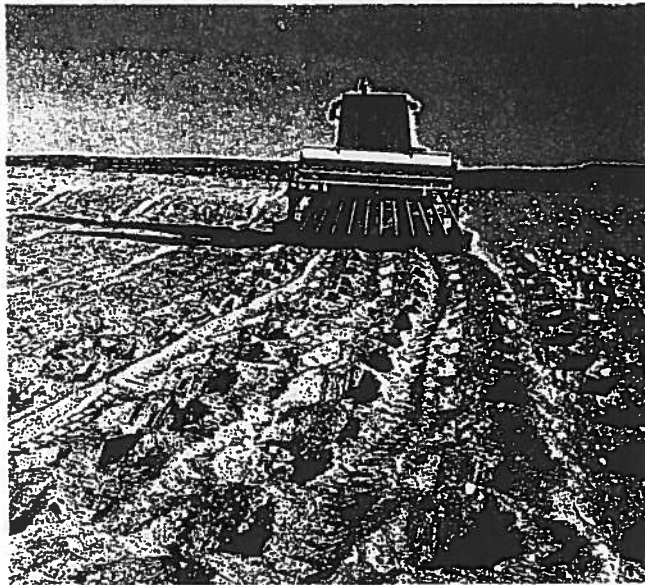
—At the Emery study area, seeding and gouging simultaneously with the gouger developed at the Missoula Equipment Development Center. December 1977.
