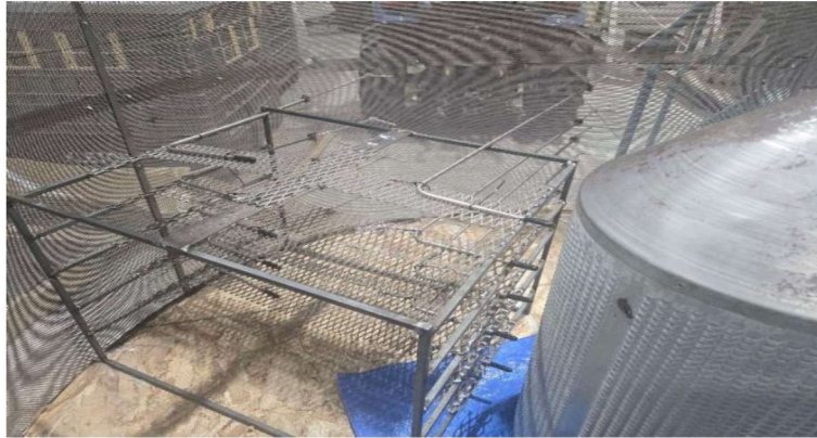
Figure 9. Pitot support frame with pitot tubes installed.
