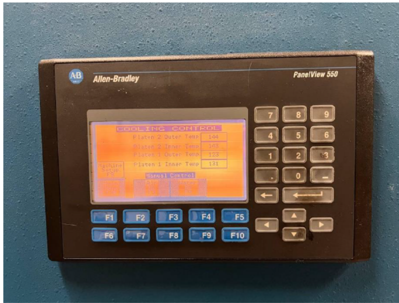
Figure 16. PanelView 550 of Wabash press showing the cooling controls
