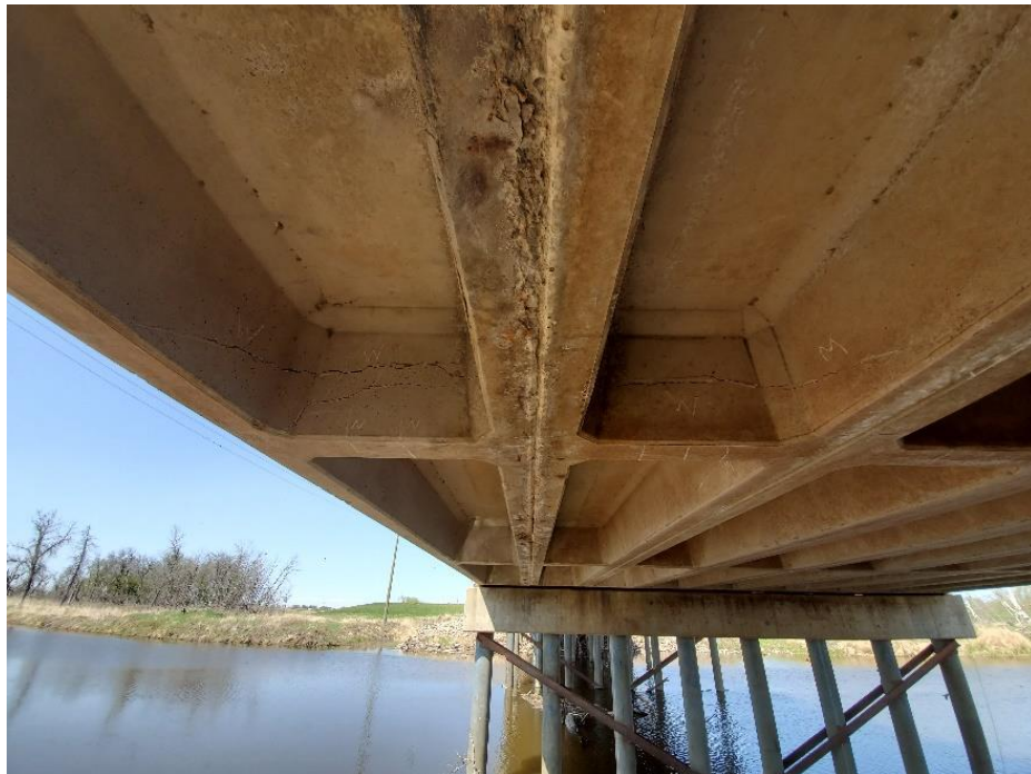
Figure 2: Wide Cracking at Post Tension Ducts in PPCC Bridge (Author's Photo, Melita Manitoba)
