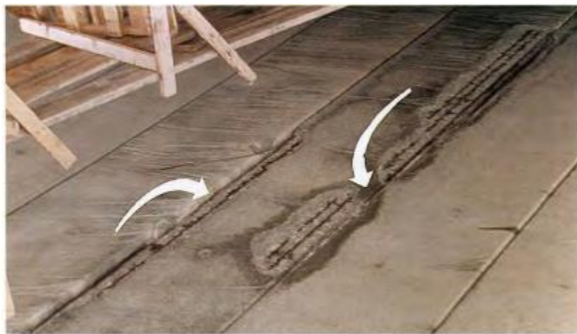
Figure 1: Corroded and Deteriorated Prestressing Strands Adjacent to Grouted Keyway ( Gulyas 1995 )
