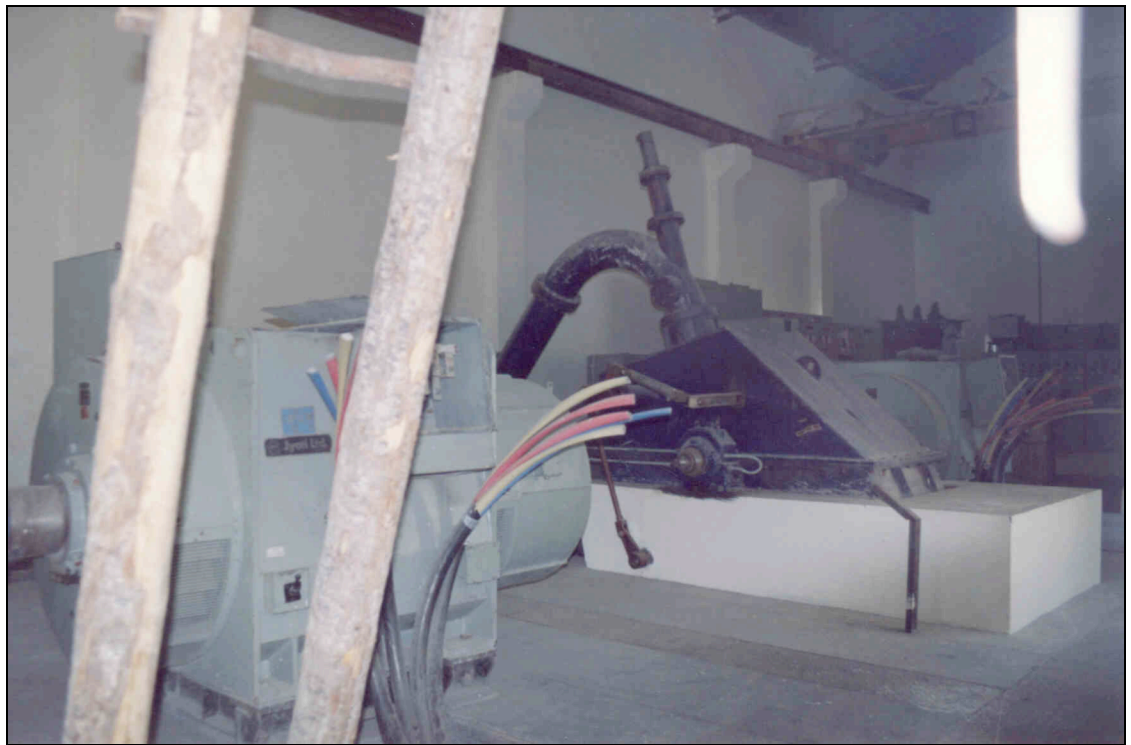
Plate 4-12: Jumma hydro plant interior.
