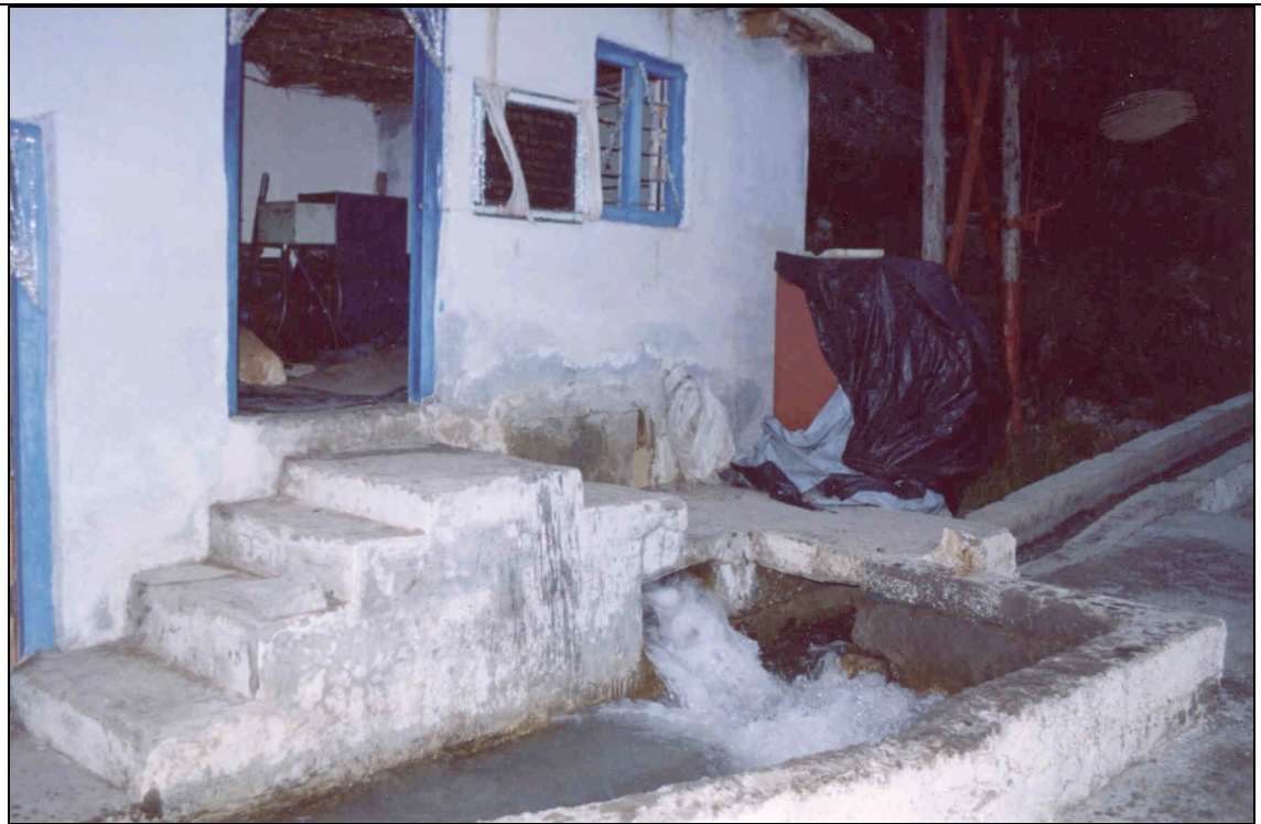
Plate 4-3: Exterior of Malari Powerhouse showing outflow.
