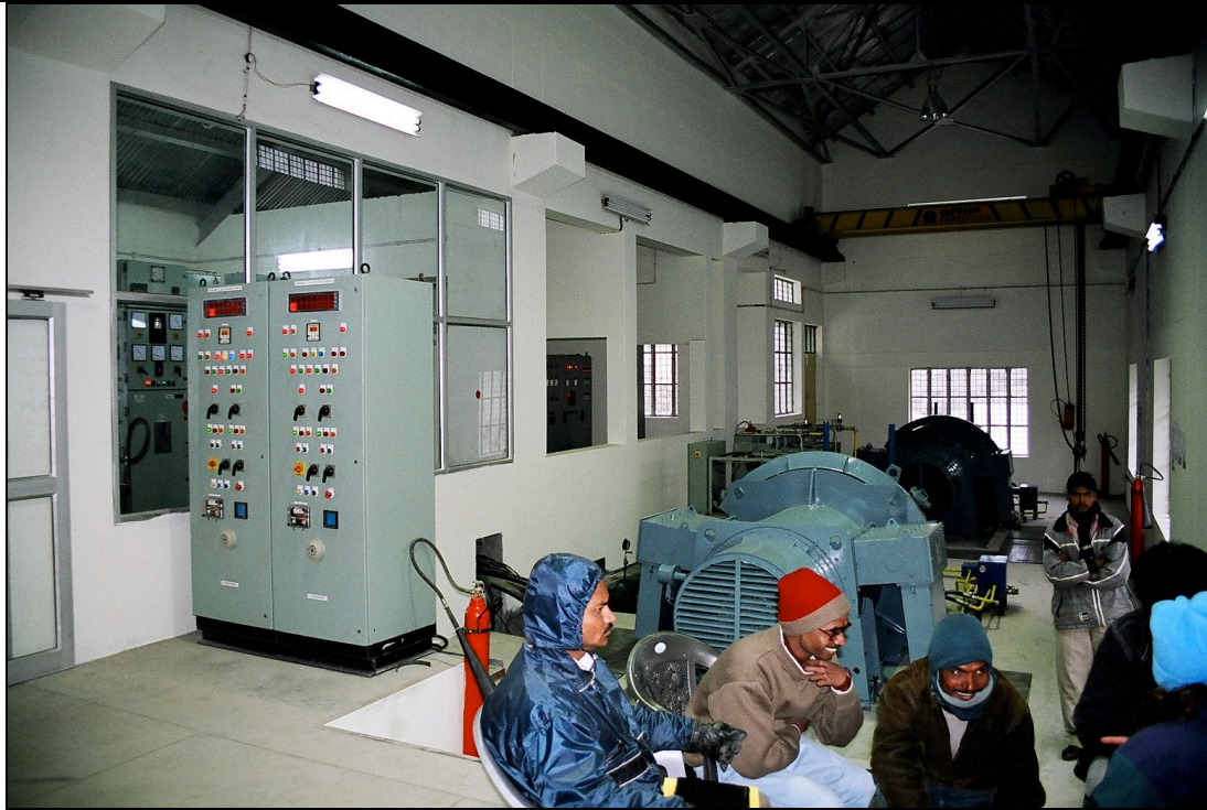
Plate 4-9: Interior of Badrinath powerhouse.
