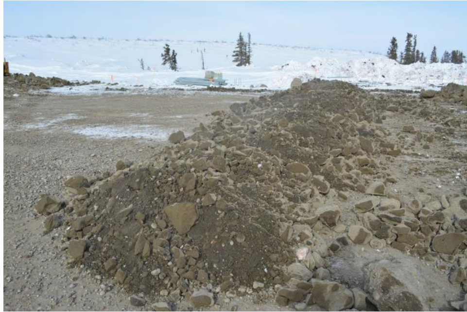
Fig. 2.3. Frozen soil used from borrow source pit (Pit 174) during embankment construction at KM 82+380.
