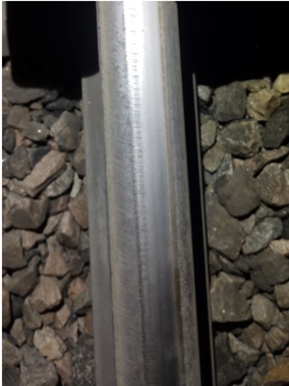
(a) Pre-grind rail face.
