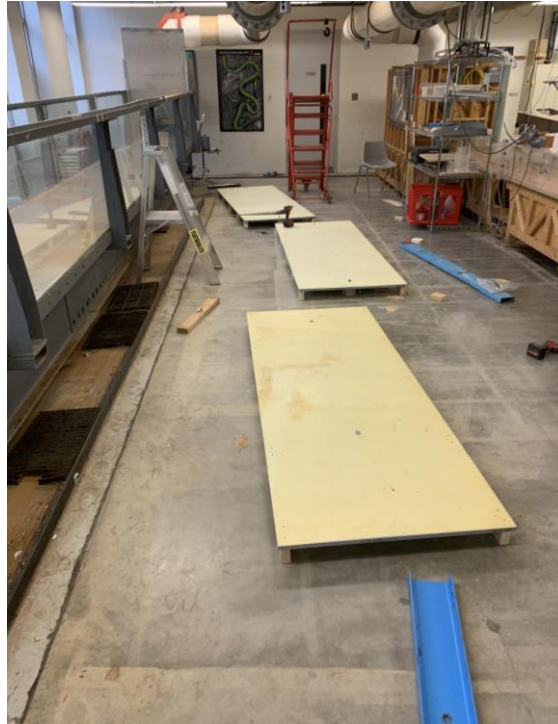
Figure 18: Subfloor HDO panels and C-channel girders (attached for weight) pictured during construction
