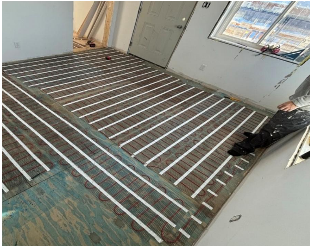
Figure 4.13: Radiant floor installation by Wikiwin students in their new passive solar design
