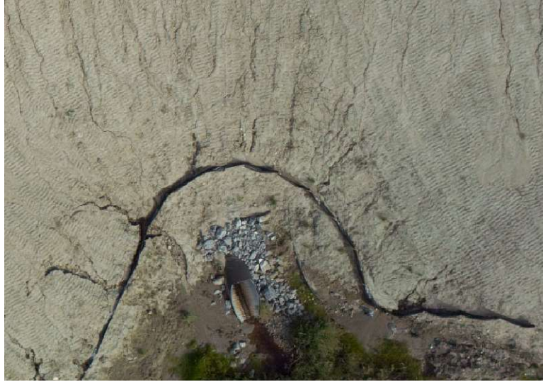
Fig. 3-5. Aerial shot of slope cracking above culverts.
