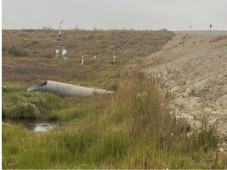
Fig. 3-10. Broken culvert at the upstream side of the embankment.
