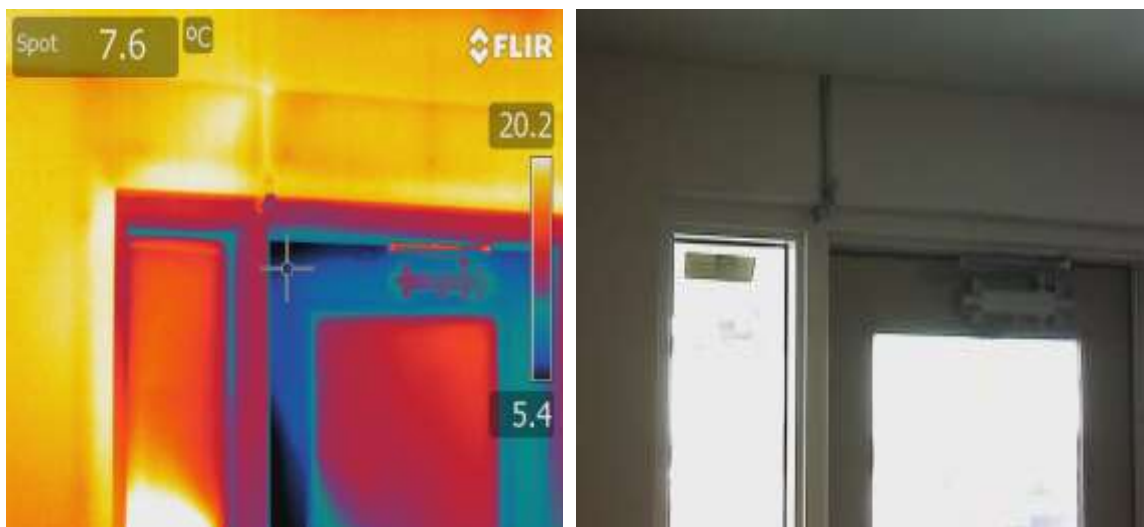
Figure 34 Air leakage through the top of the door
