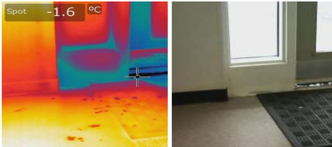
Figure 33 Air leakage below a door cools the surface of the surrounding floor
