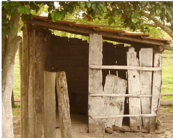
Figure 4.11 Latrine used by local residents in the San Juan del Ñeembucú district.
