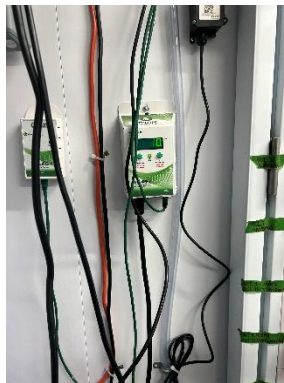
Figure 18 Titan Controls CO2 Sensor
