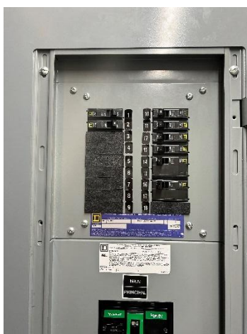
Figure 20 Electrical Panel Set-up
