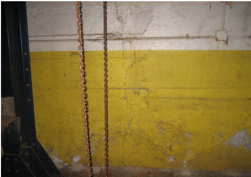
Cracked concrete wall
