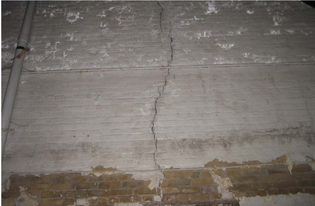
Cracked brick wall
