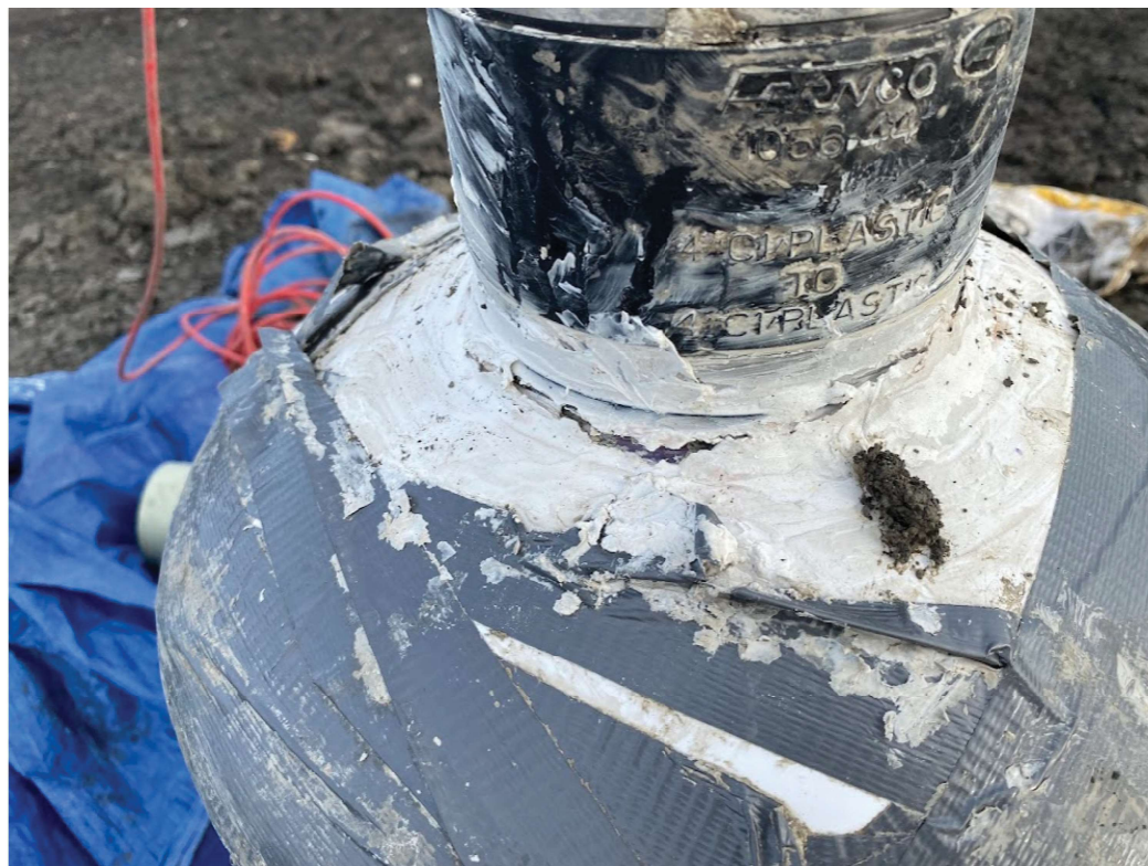
Picture 8: Leakage of Standpipe in floor test
