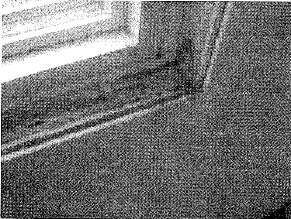
Figure 6.10: Mould on Window Sill
