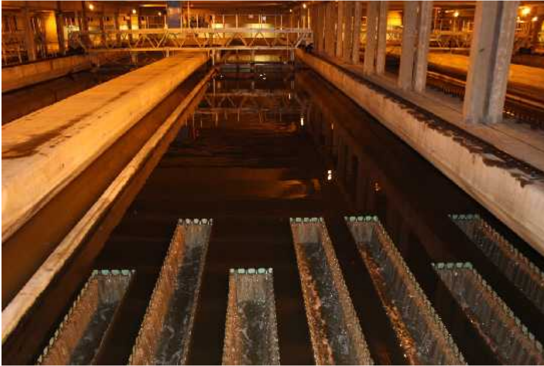
Figure 1.9 One of the 26 final clarification tanks during the secondary treatment process. Water flows from the rear to the front of the tank moving over the combed concrete teeth prior to collection and movement to UV disinfection.
