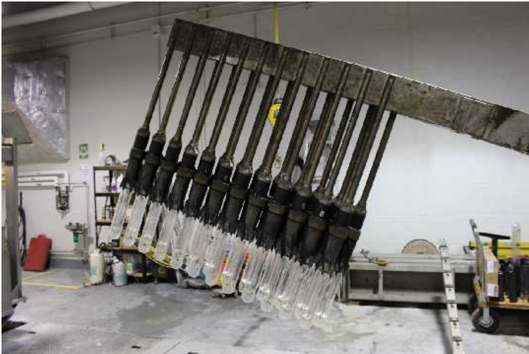
Figure 1.10 Close up view of each bank of UV bulbs used during the tertiary disinfection treatment process.
