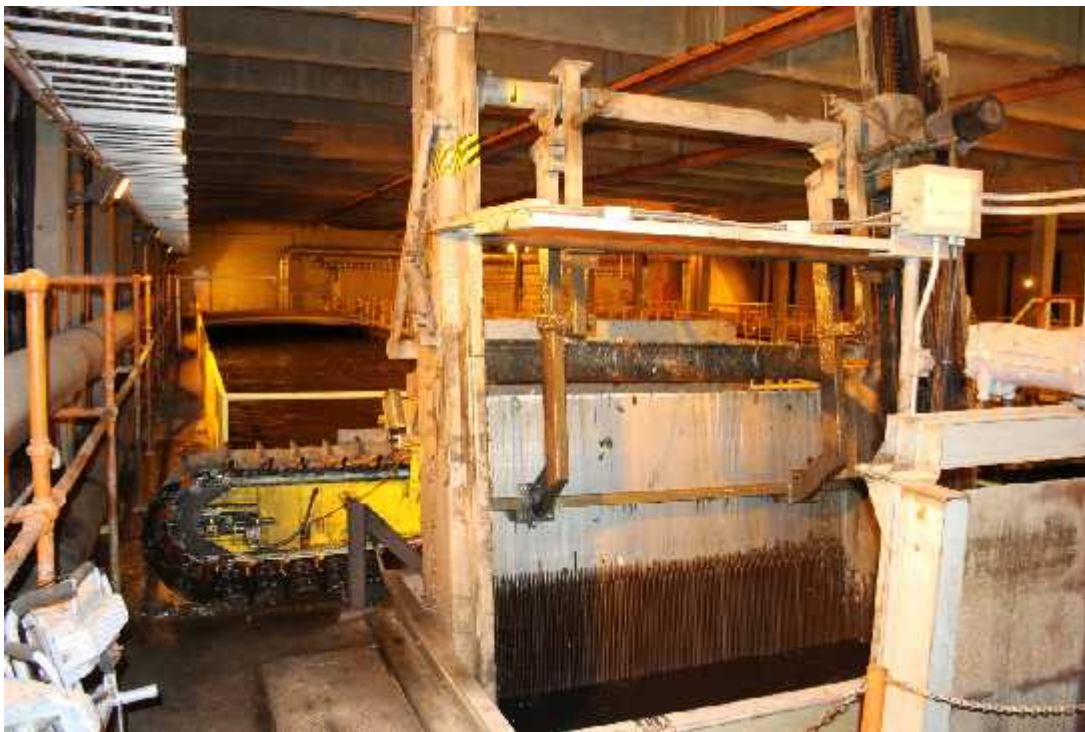
Figure 1.8 The grit house pre-aeration stage, including the holding tanks in the background, and the screeners and conveyor belt in the foreground.
