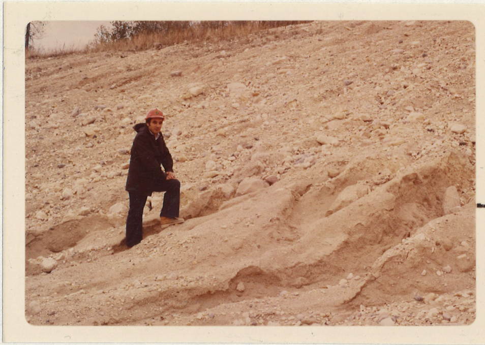
Photo #22: This slope was graded to an angle of about 18 degrees (30%) four years prior to the picture, but no vegetation cover was established. Erosion has exposed rocks on the surface and formed gullies measuring 18 to 24 inches deep.
