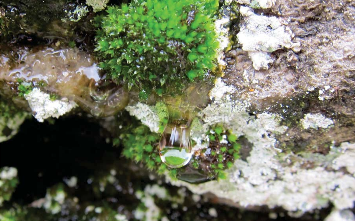
Figure 9.05: Ground water drips from moss in a crack in the Lily Pond rock wall.
