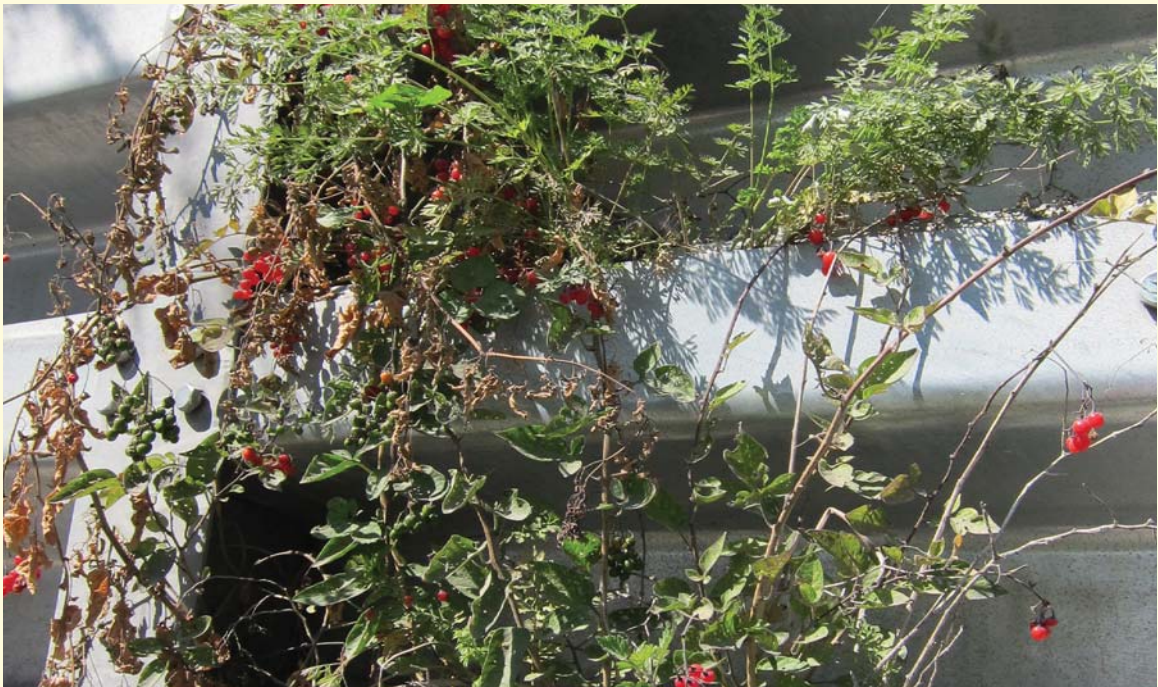
Figure 8.07: Unplanned colonisation of a steel wall by plants on a southern facing street-side retaining wall, Toronto. Note species of yarrow, nightshade and grasses.
