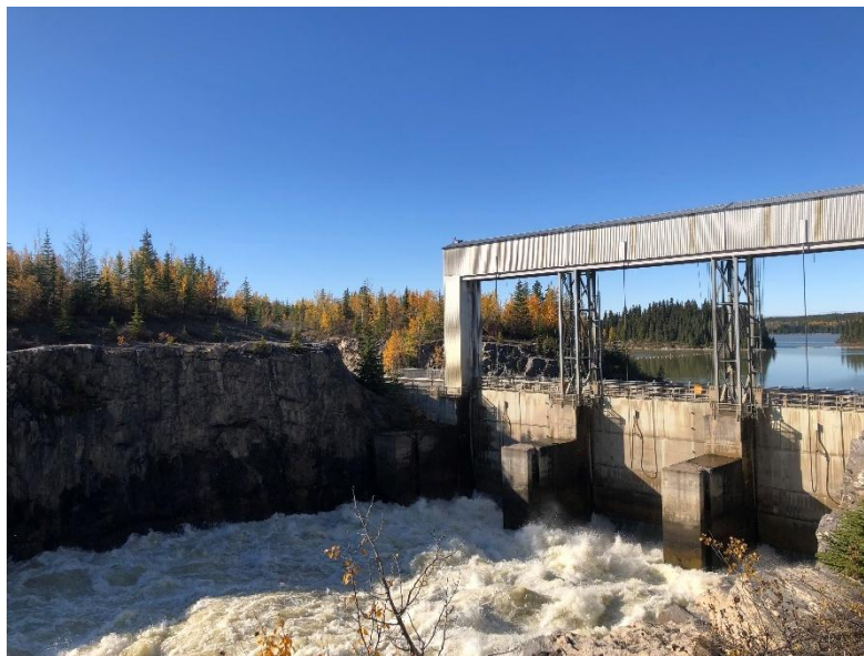
Notigi Control Structure on the Churchill River Diversion captured by Bobbie Mangeli in October 2022.
