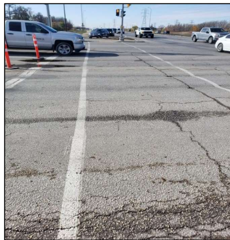
Figure 1.1 Rutting at an intersection in Winnipeg
