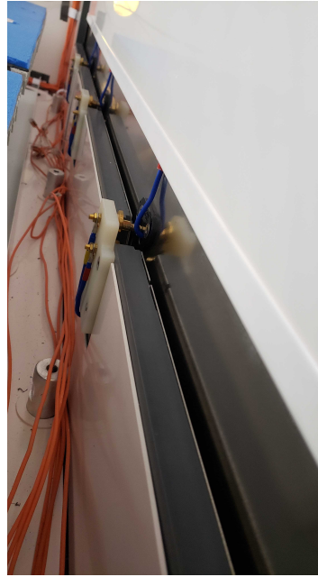
Figure 5.20: Layer 5 gap inside the room once the door is closed. The gap is about \sim 5 mm.
