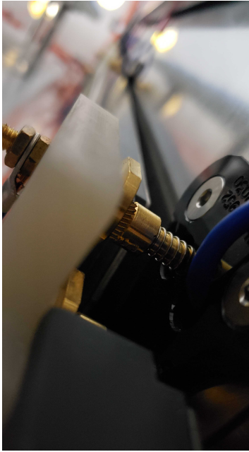
Figure 5.19: Layer 5 distributed degaussing connection not connecting when the door is closed.
