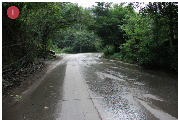
The main access route connecting the site to the residential areas above is a steep and winding dilapidated two-lane road.
