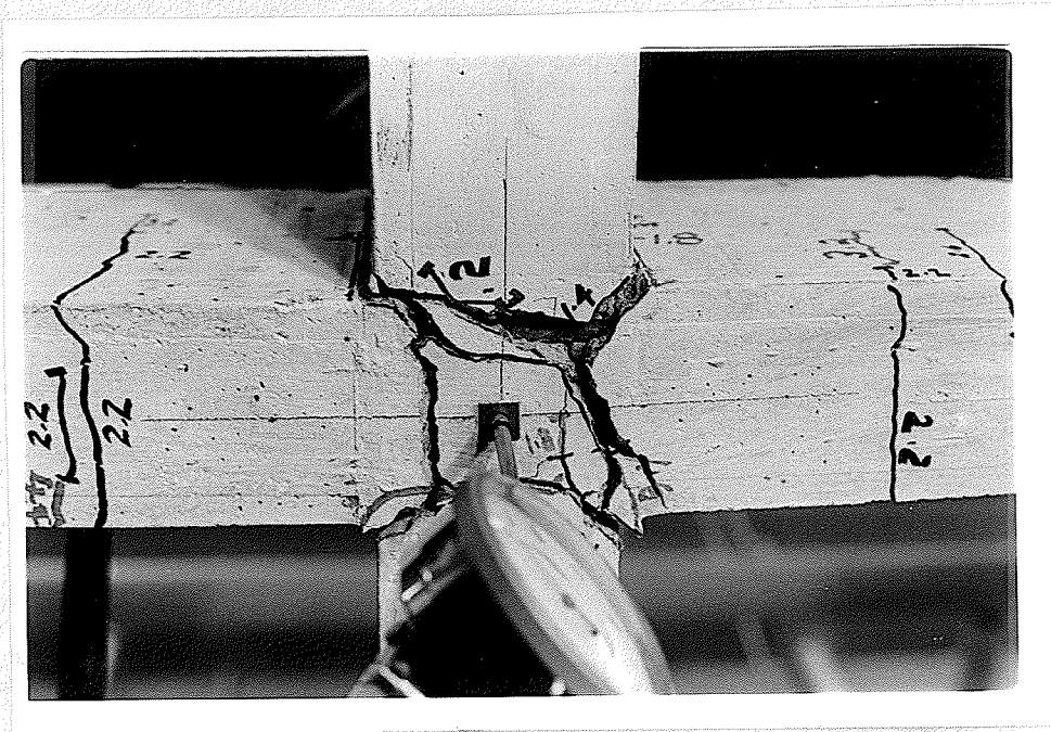
Figure 30. Crack Development Directly Under Load.
