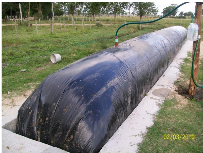
Figure 1.3. Biogas installation with tubular PVC membrane bags in Costa Rica.
