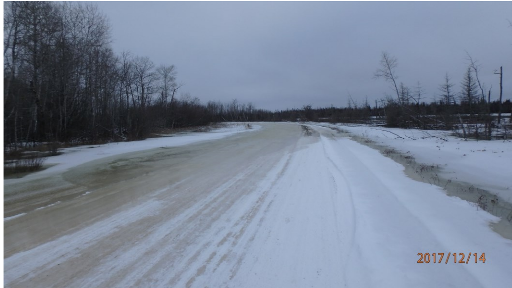
Figure 2.30. Overtopping of PR 513 on December 14, 2017 caused by ice-affected staging.
