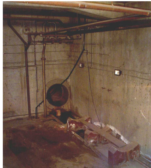
▲ F72 | BASEMENT 1 | PIPING
