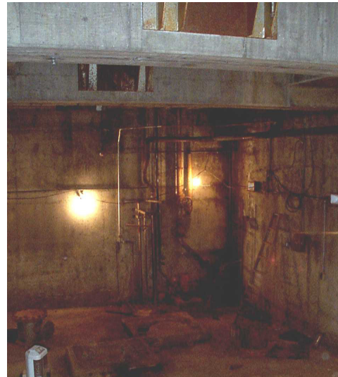
▲ F70 | BASEMENT 2 | PIPING
