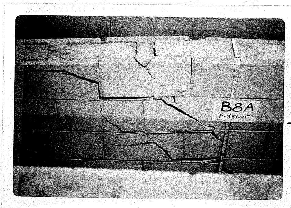
FIG. 55 SHEAR FAILURE IN BEAM 8A
