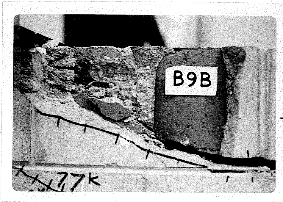
FIG. 68 CLOSEUP OF SHEAR CRACK AND CRUSHED CONCRETE IN TOP OF BEAM 9B
