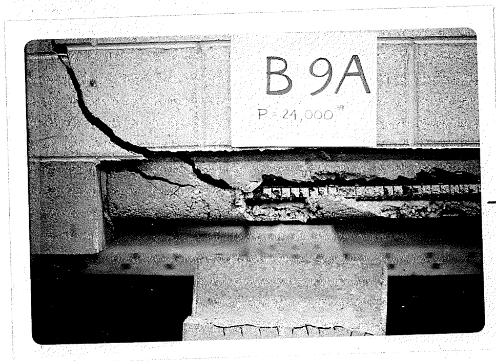
FIG. 57 CLOSEUP OF SHEAR CRACK IN BEAM 9A.
