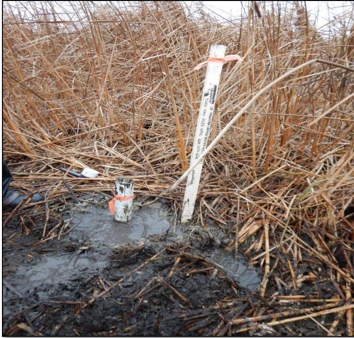
Figure 3.6 - A completed GP5 well installation. A plastic pipe with a lid sticking out of the ground. Contact person information were written on the white stick (beside the pipe).
