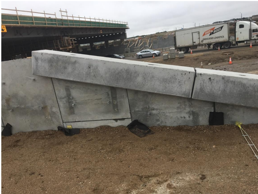
Figure A-12 – Elevation of Compacted Granular Fill Behind North Wall on June 2, 2018
