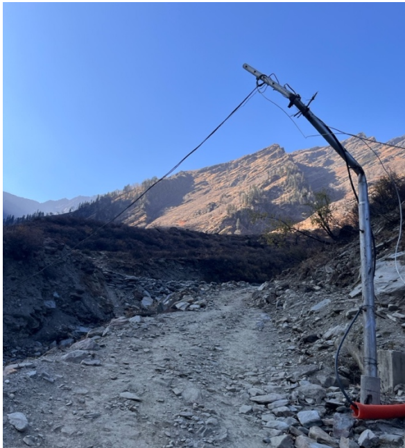
Beaskund Top Broken Transmission Line Poles
