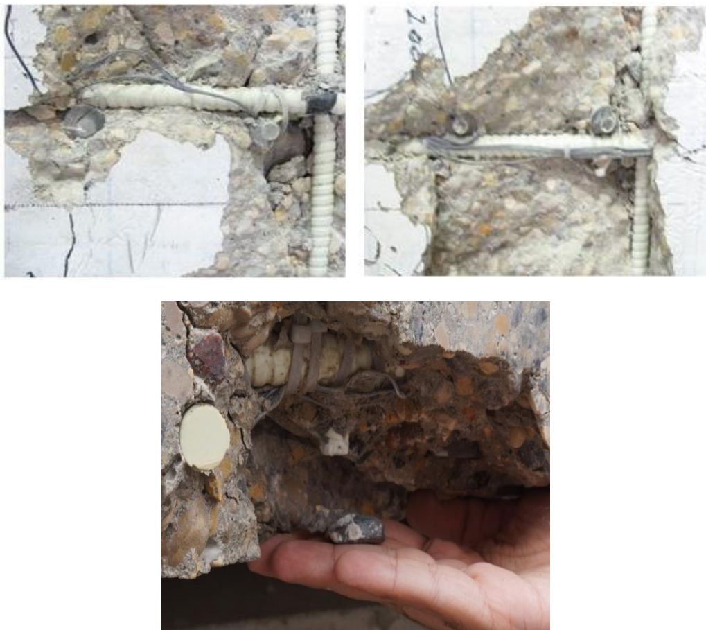
Figure 4.16: Damaged heads for the GFRP shear studs
